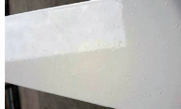
Above: Here, you can see defects experienced in the powder coating finish from the oven residues.
