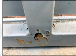
Figure 1. Corrosion Around Weld Areas of Steel Fence Structure
