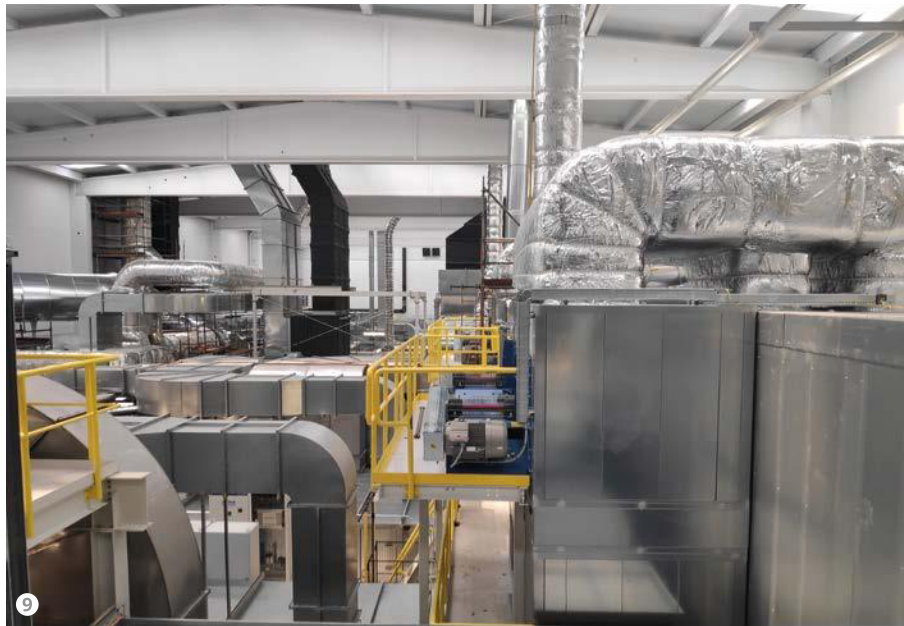
Figure 9: One of the technical levels of Mapsa’s painting installation.
