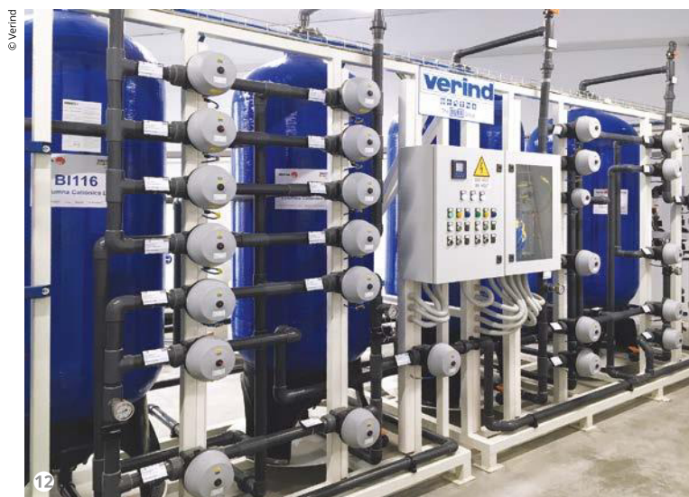
Figure 12: Duplex automatic demineralization system.
