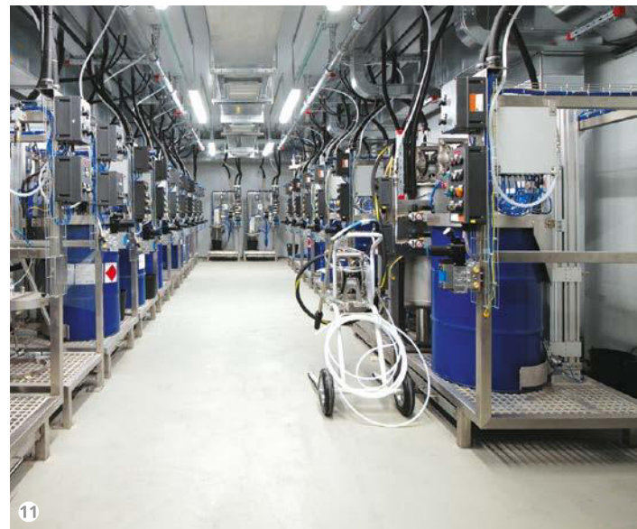
Figure 11: Paint mix room box with paint pumping unit for BC and complete with Dürr pumps and controls.
