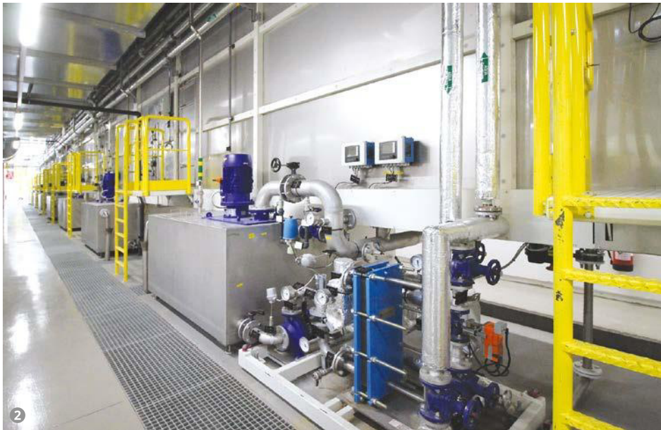
Figure 2: The spray pre-treatment tunnel.
