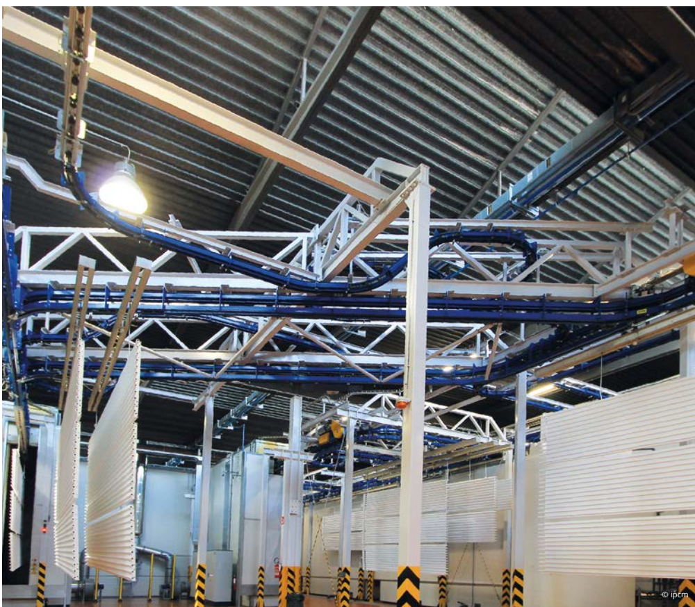
The curing oven.
