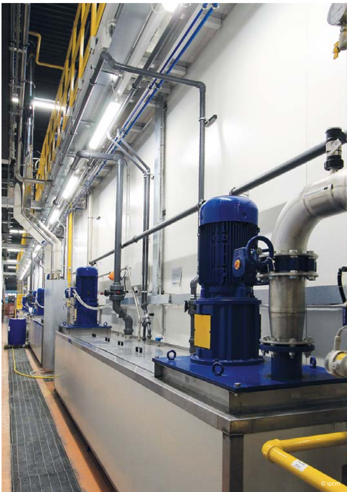
The large pre-treatment tunnel.
