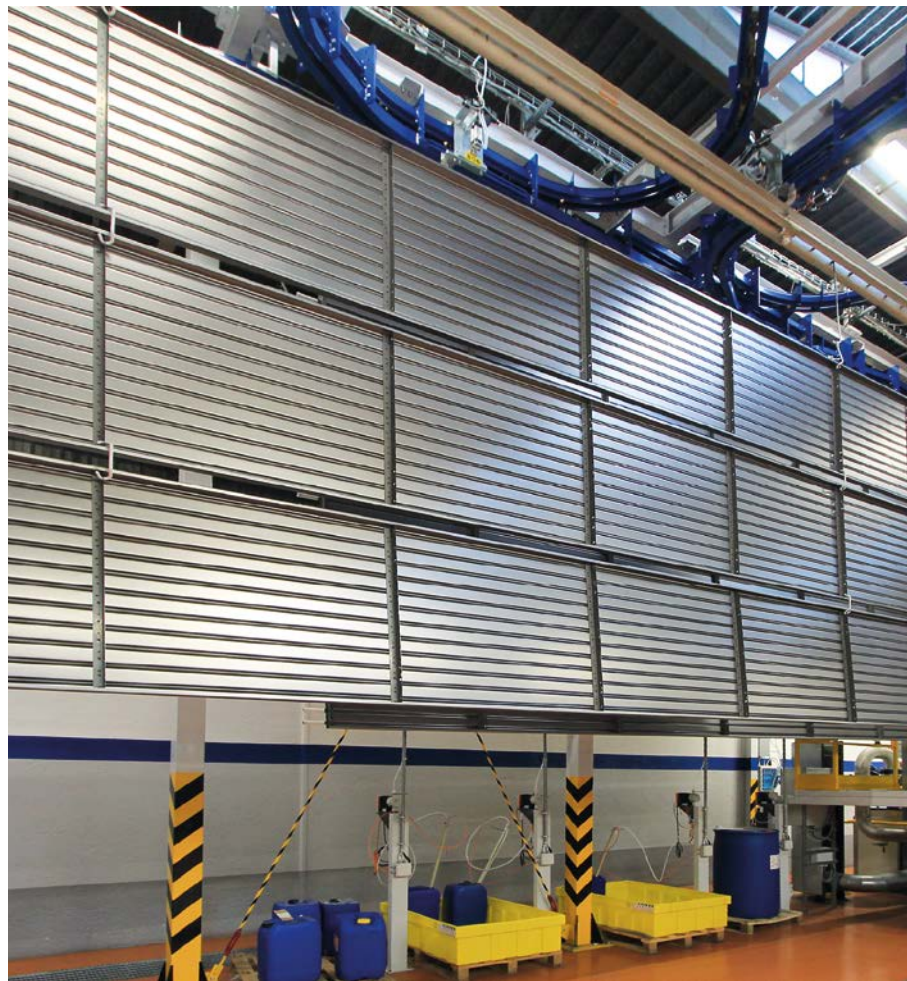
Radiant plates entering the pre-treatment tunnel.
