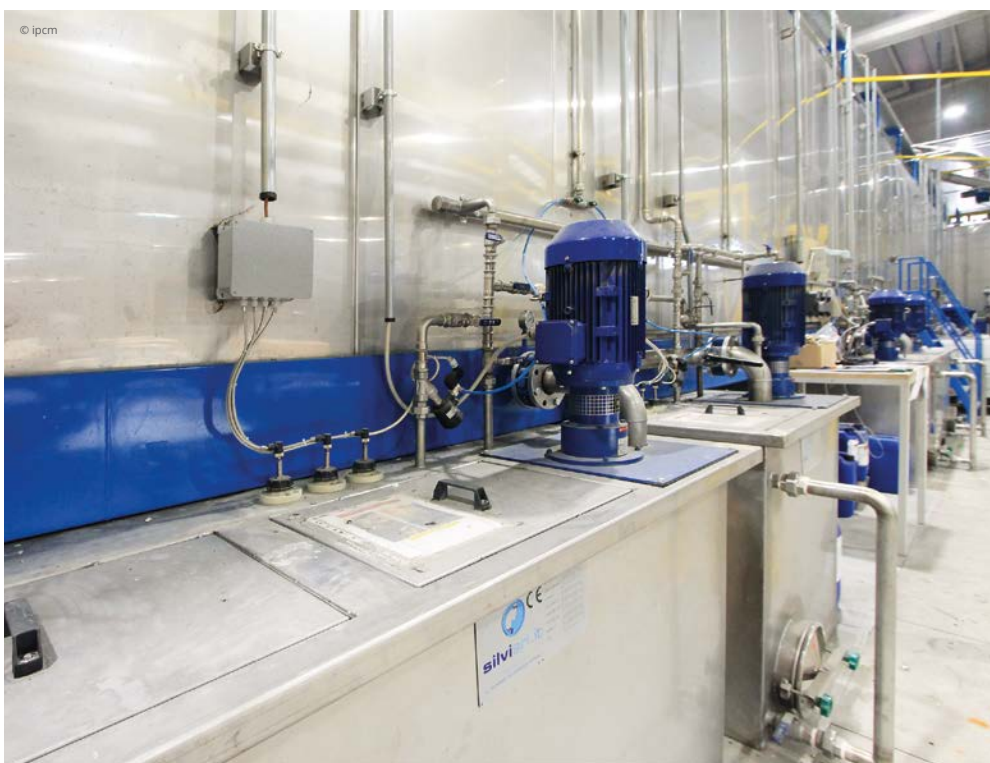
Top left: The loading station.
