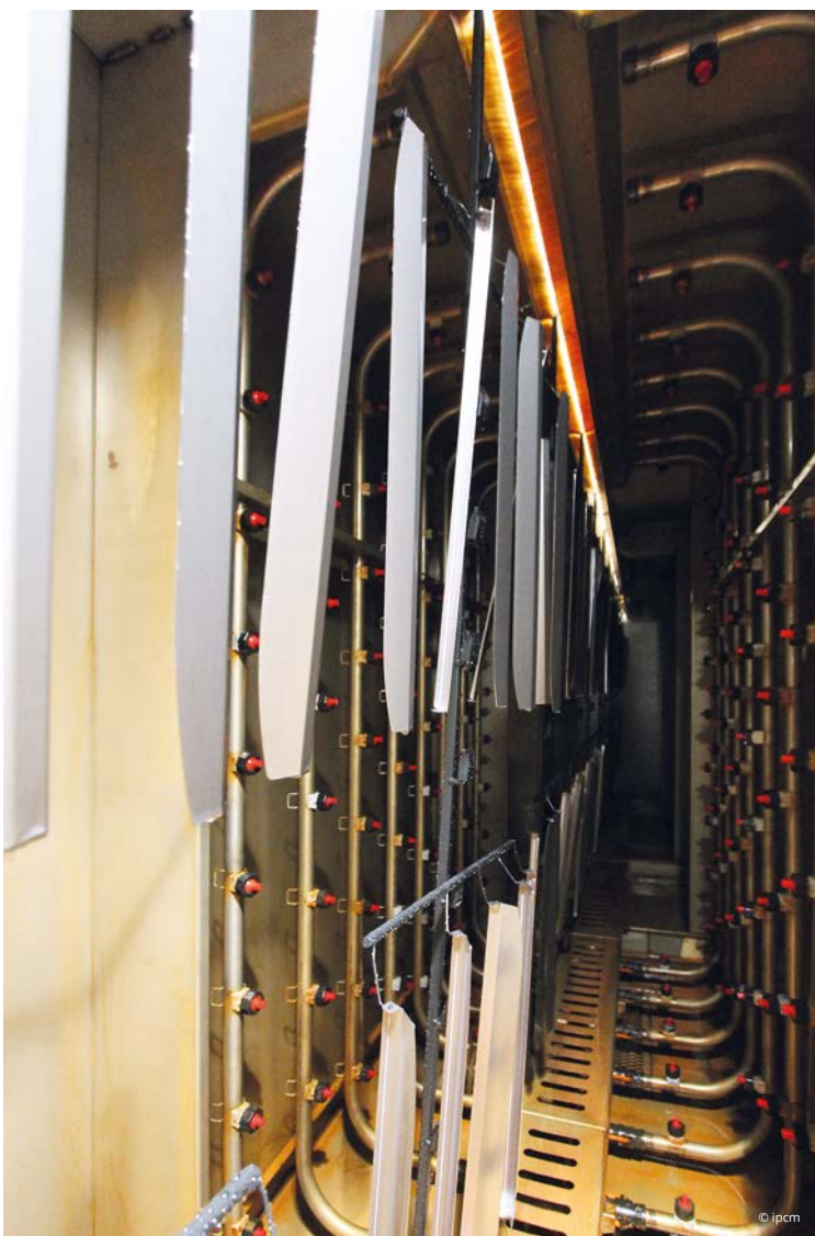
The inside of the pretreatment tunnel.
