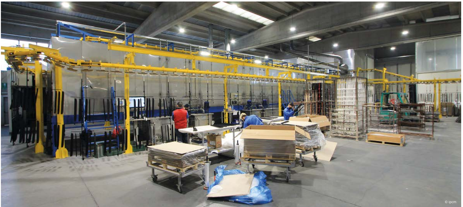
Overview of the new powder coating installation designed and installed by Silvi Srl.
