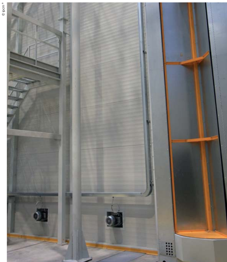
The fans are positioned at floor level of the oven.
