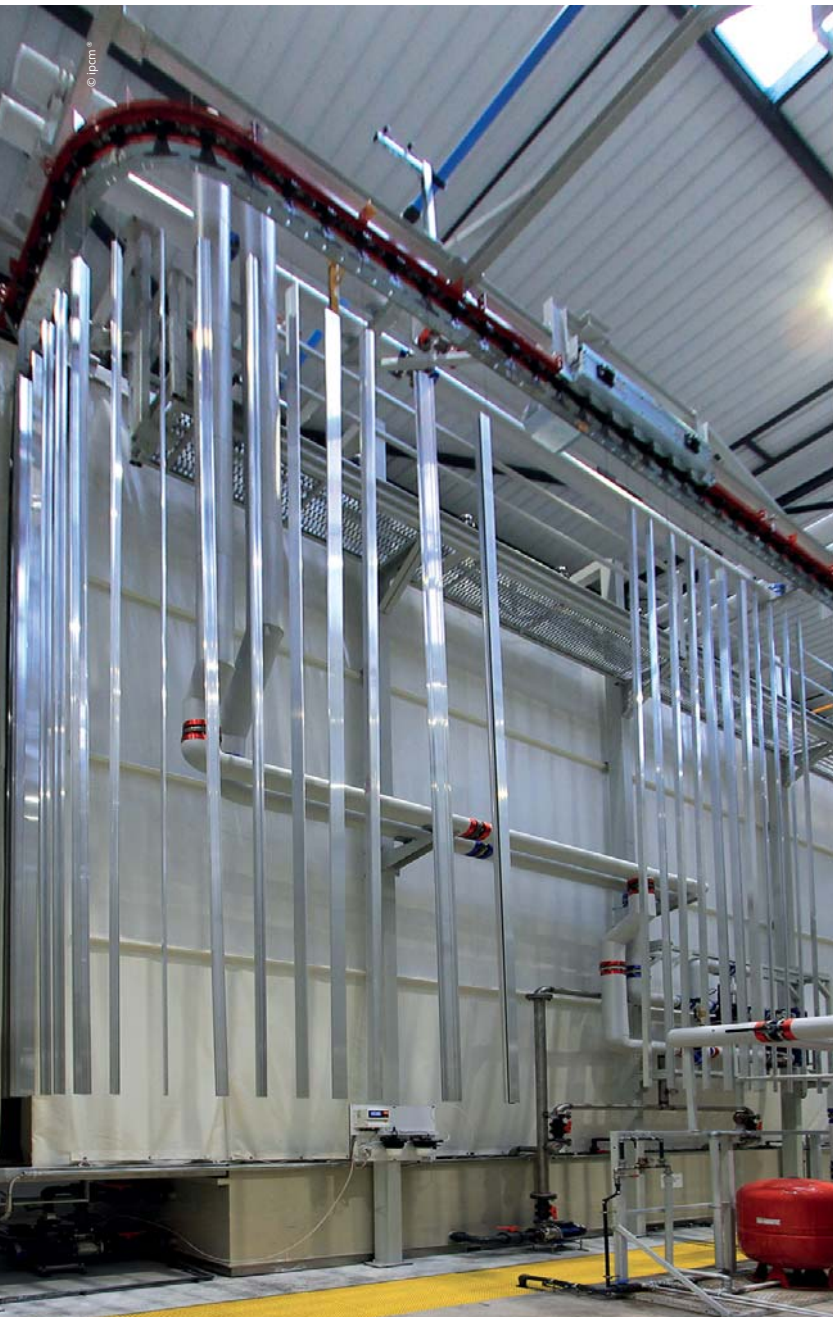
The pre-treatment tunnel.
