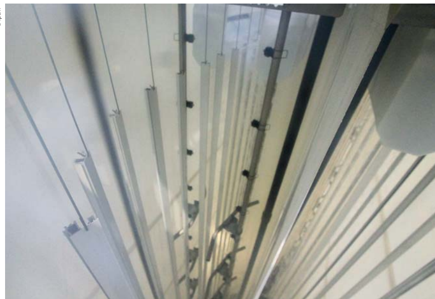
Internal view of the pre-treatment tunnel.
