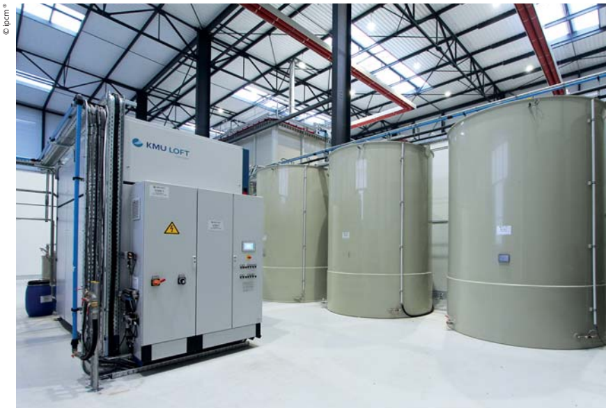
The vacuum evaporator of the water treatment plant.
